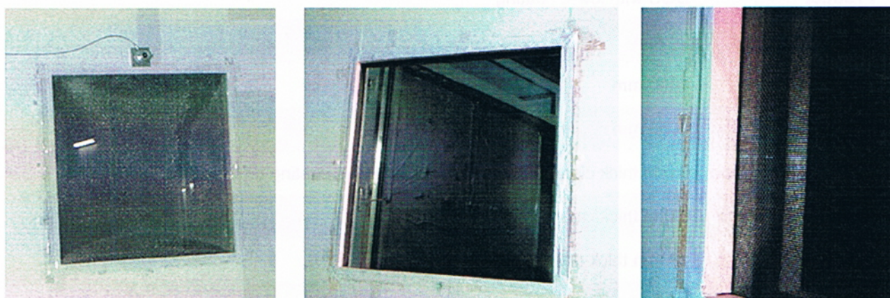
Figure 3. Photos of the installation. Left: view from outdoor side; middle: view from indoor side; right: zoom-in view of the edge mask at the perimeter (the specimen is on the left)
